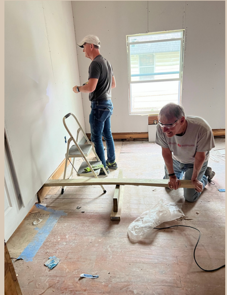
DAVE AND JIM HANGING DRYWALL (DAVE WAS VERY PROUD OF HIS DRYWALL LEVEL INVENTION)
