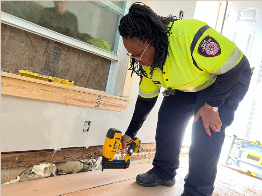
HELEN PUTTING DOWN FLOORS - SHE HAD TO JOIN IN ON THE FUN!
